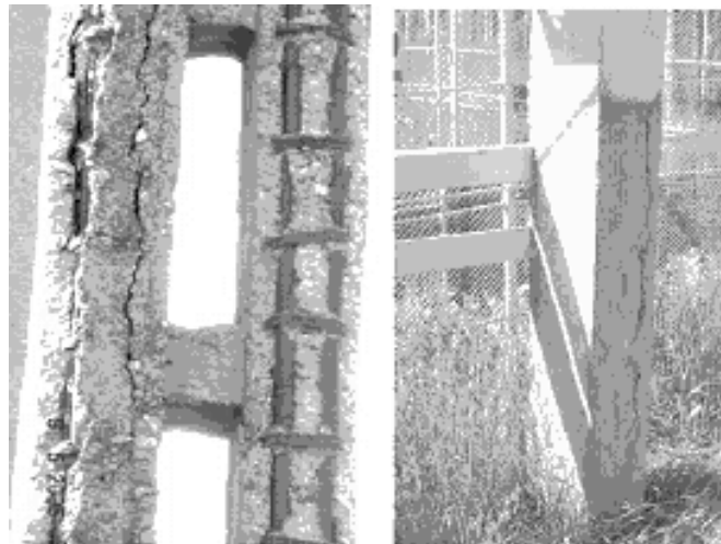
Fig. 16 – Steel concrete support elements degradation that are operating in high electromagnetic field.
